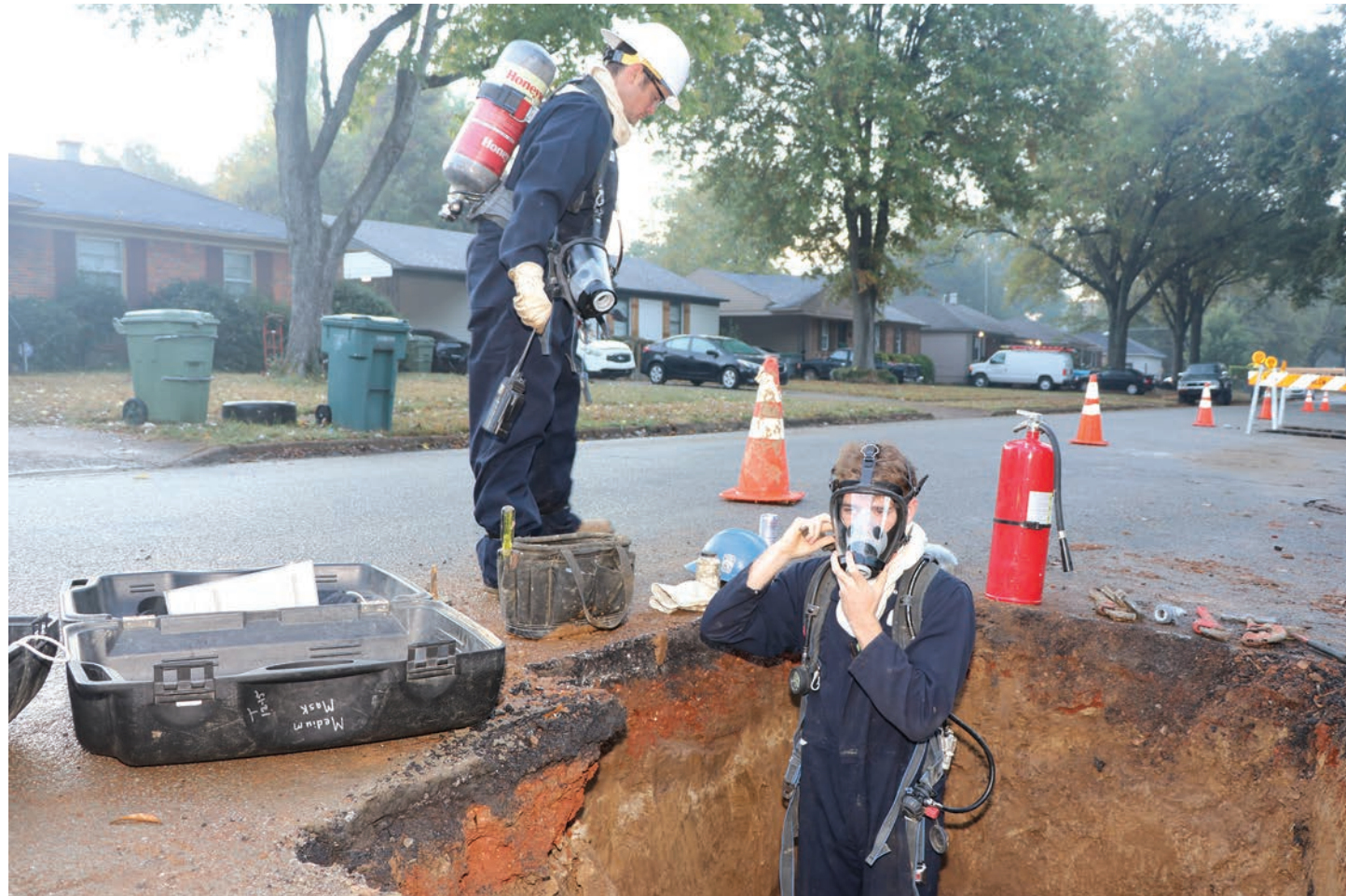
A gas worker wears a self-contained breathing apparatus as he and a co-worker set up to make repairs on a gas line. A fire extinguisher sits nearby if needed.
