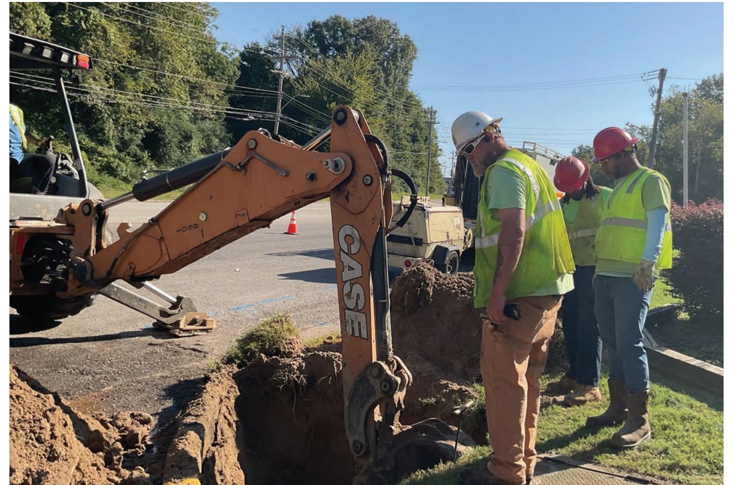
A backhoe operator carefully digs around the existing utility service lines as he replaces a water valve.
