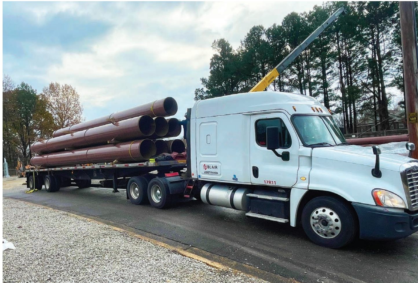
A driver delivers the first 24" high-pressure gas transmission pipeline load for the $30 million Weaver-Gill modernization project.
