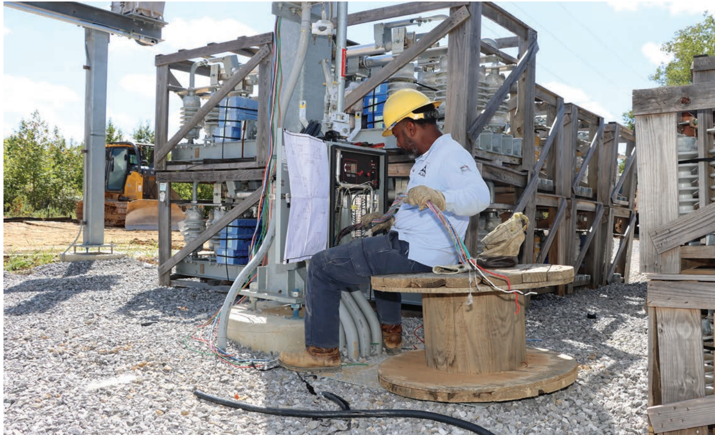
A construction crew member follows the blueprint for a circuit breaker at the brand-new $23.6 million Collierville substation site, which is underway. Once the substation goes online, it will improve reliability and reduce the electric loads in southeast Collierville and Shelby County.
