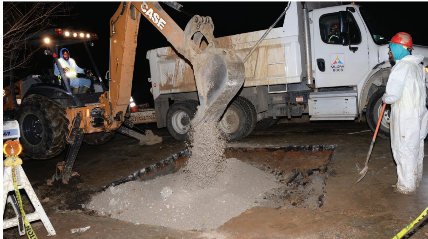
Once a water line project is completed, a Paving & Concrete Restoration crew returns to repair the street before morning rush hour.
