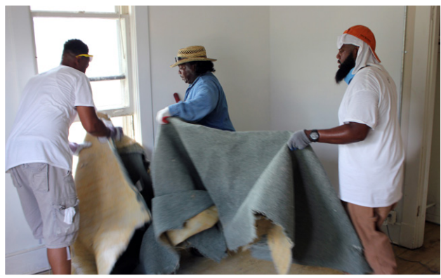
Pulling up several rooms of carpeting at Grace House was dusty business. Hauling dusty, dirty carpet are (l-r) Steering Committee members Brandon Still , Accts. Payable, and Derrick Smith , Gas Transm. Svc., along with Chris Cleaves , Transf. Elec. Motor Shop.
